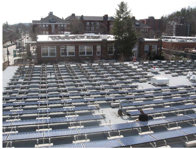
Solar panels cover the roofs of the Sanders Administration Building and Anthony Student Service Center.
